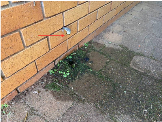
Hotwater system overflow falling next to the house in the southern side.
