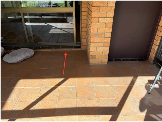
Concrete porch obstructing the termite shield inspection zone.
